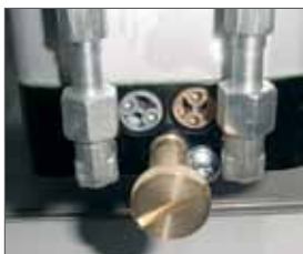
By pass valves
